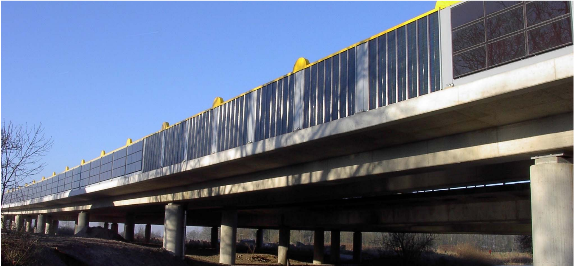
Photovoltaic noise barriers in Emden
